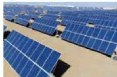
OFF-GRID PV station
